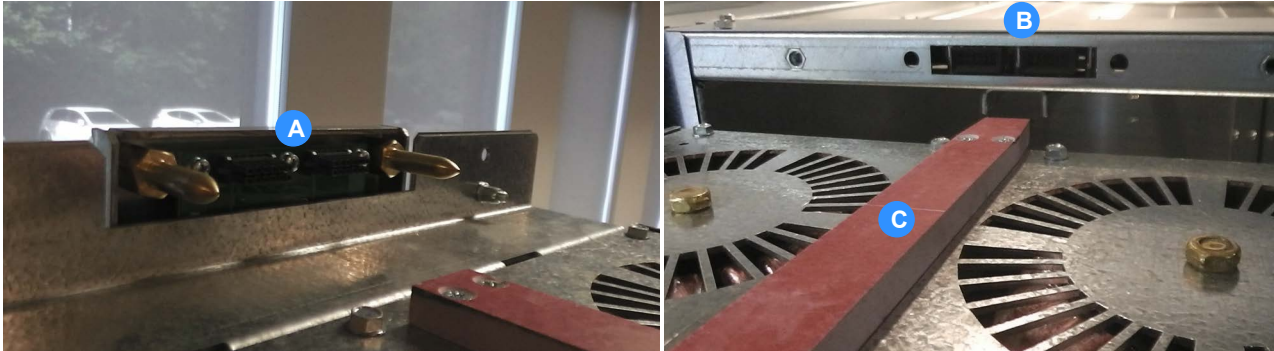
Figure 2.21 UPS module parallel bus connectors
